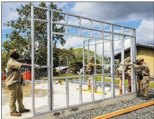
Engineers from the Australian Army, British Army and PNGDF work together at a construction site during Exercise Puk Puk at Goldie River Training Depot
